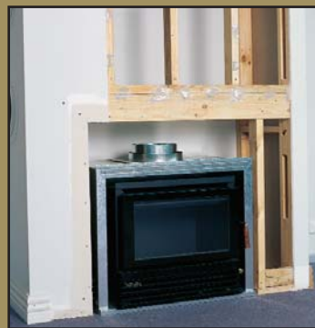
Heater fitted to Zero Clearance box
